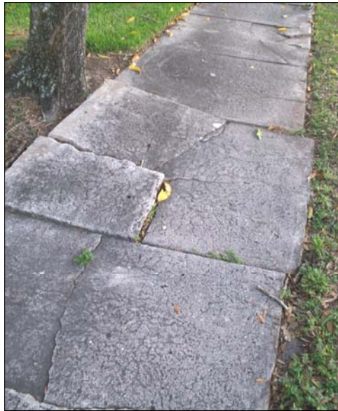
Buckled Sidewalks due to Tree Roots
